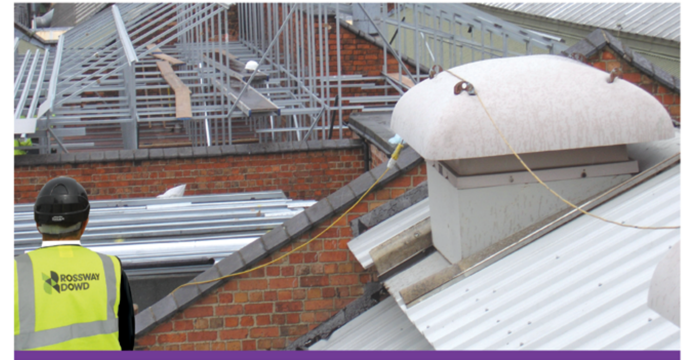
Rossway roof dilapidation assessment
