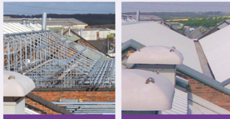
Brush Electrical before and after, Loughborough
